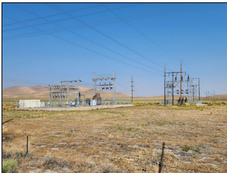
Figure 3: Existing HEC Substation located close to planned plant site.
