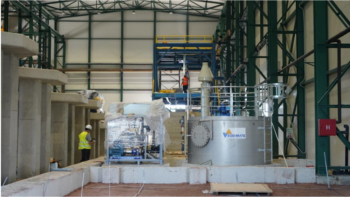
Figure 8: Lime system, flotation building, July 2023
