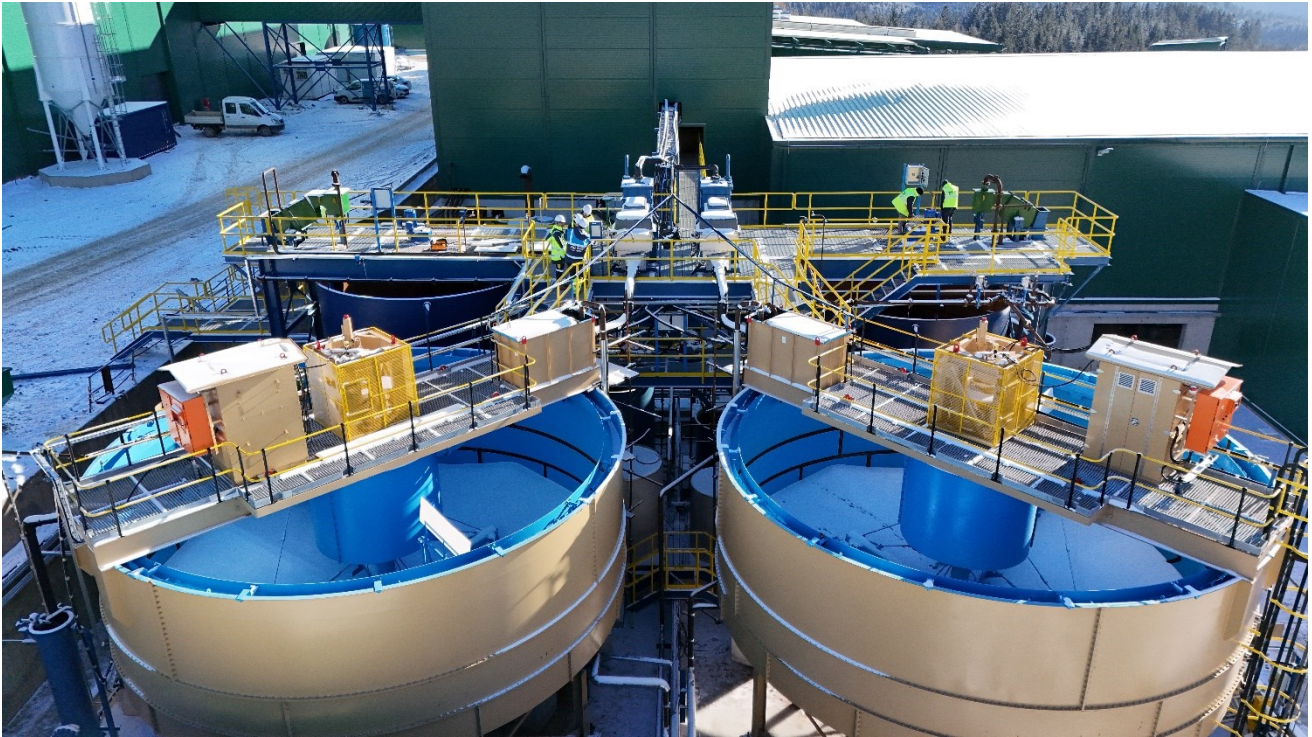
Figure 12: Thickeners (lead and zinc), January 2024
