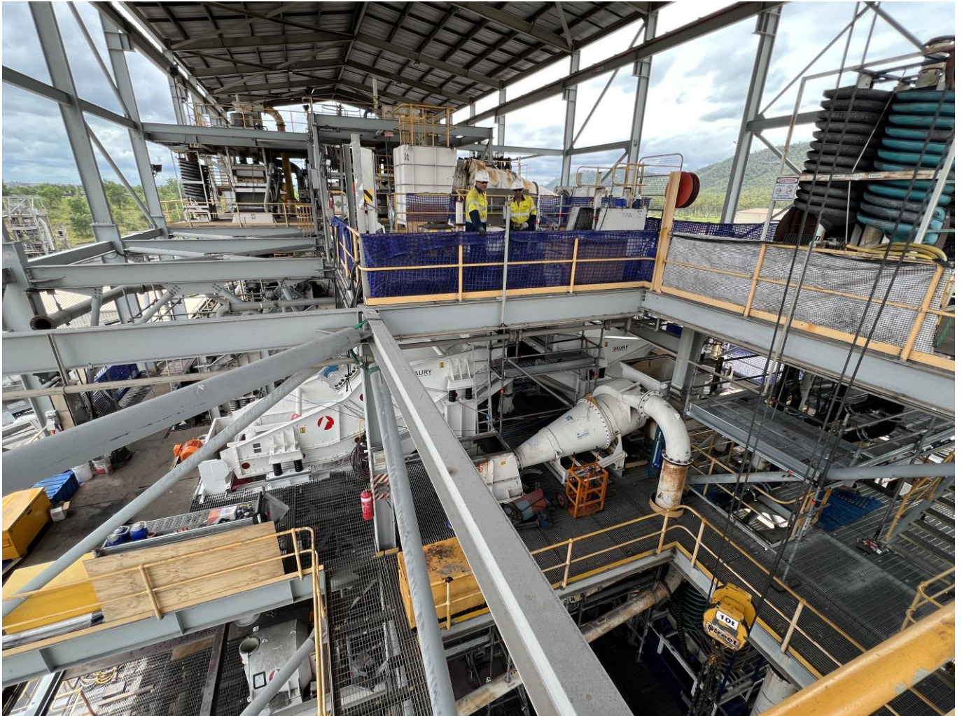
Figure 2. Refurbished cyclones and screens for Module 1 being fitted in the Burton CHPP
