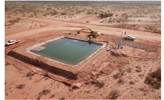
Figure 4. Turkeys nest for construction water
