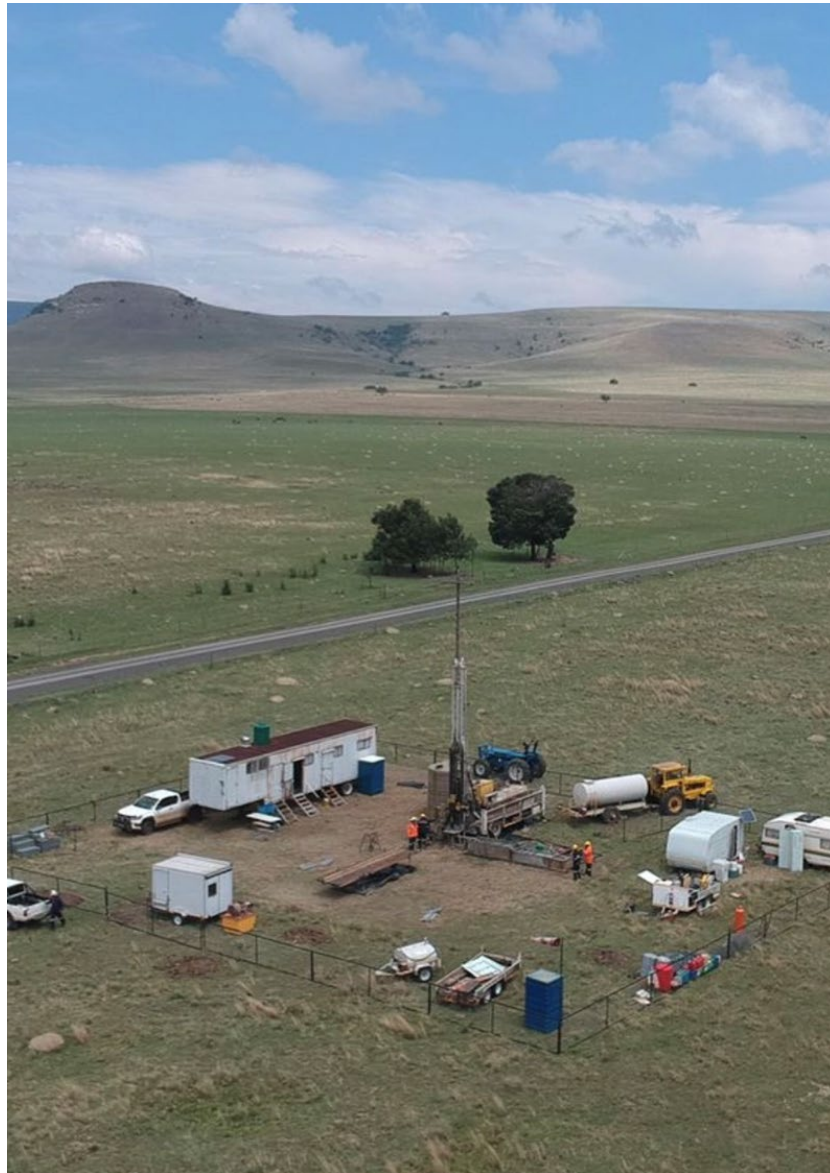
Figure 3 - Core well 270-06C being drilled in the southern most region of the Company's granted rights
