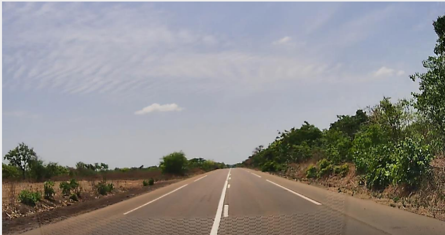
Typical road condition - Tingrela area, Côte d'Ivoire
