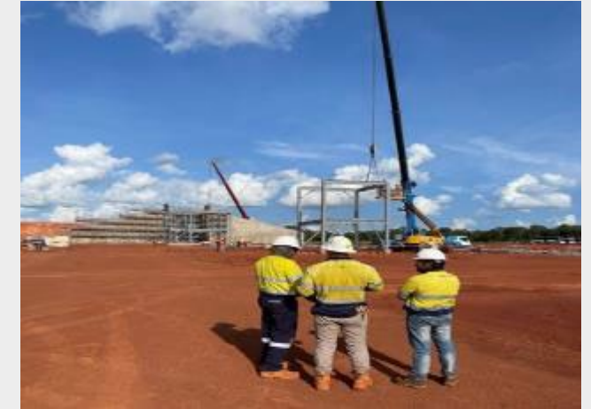
Structure for primary crusher discharge
