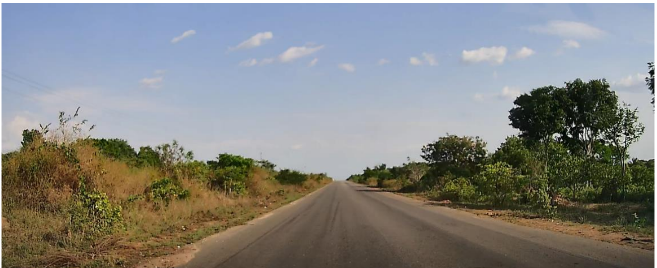
Indicative Road Condition at Seguela between site and Port of San Pedro.
