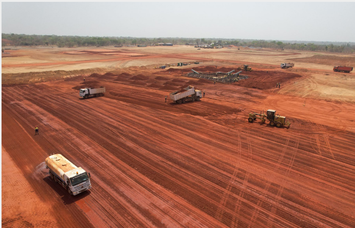
Process plant site: clay removal and backfill Next: prepare foundations of mag circuit and thickeners
