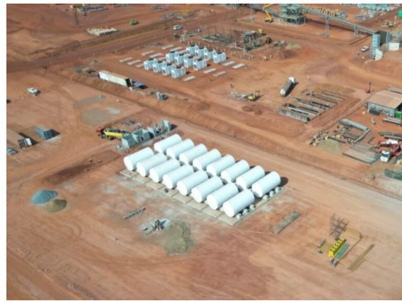
Figure 9: Fuel storage and power plant
