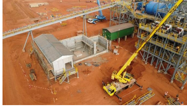
Figure 13: Elec. Switch room/transformer house
