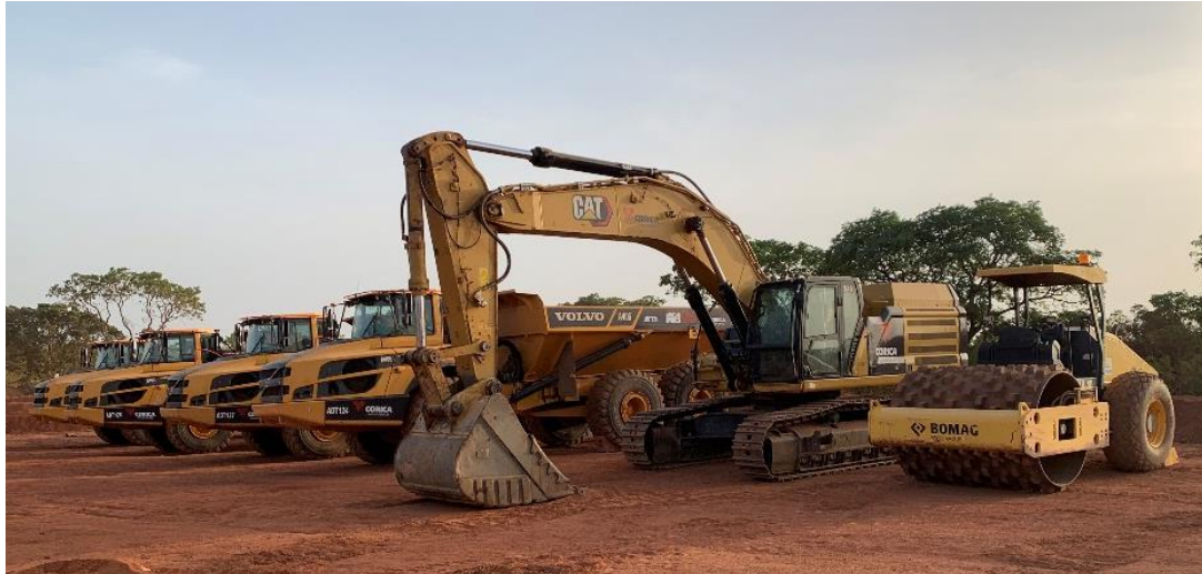
Corica's early works fleet (Volvo ADT's and Cat excavators). Long term fleet is yet to arrive and includes CAT6030s excavators coupled with CAT777 trucks
