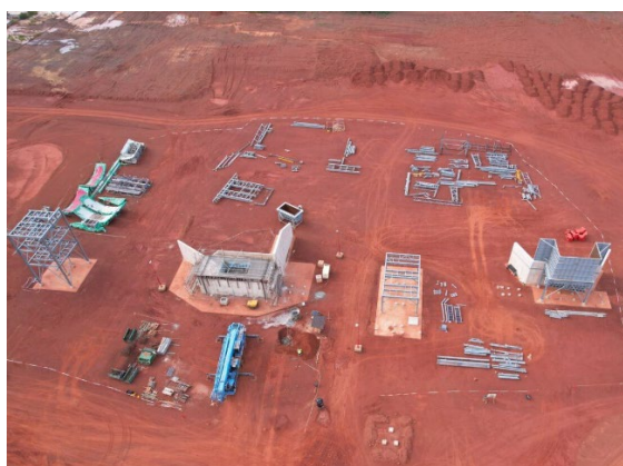
Image 5 - Fine ore bin and reclaim area
