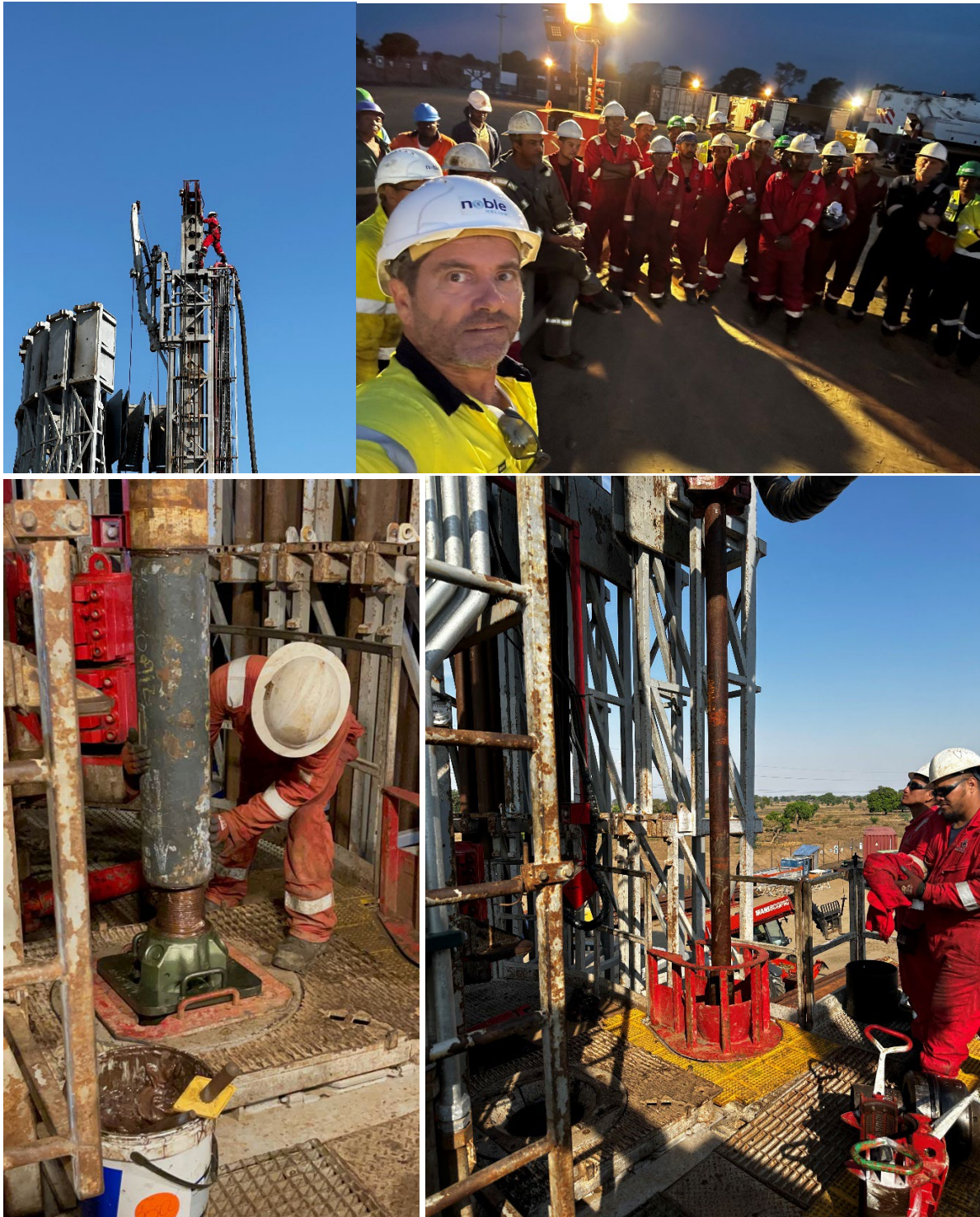
Clockwise from top left: Last-minute checks of the crown block; Pre-spud meeting with the full drilling team; Setting up drill string in the mouse hole; Attaching the first drill bit to the Mbelele-1 BHA (Bottom Hole Assembly), in preparation for spud.
