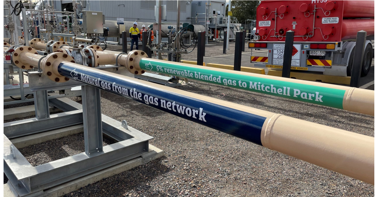
The HypSA Project in Tonsley, South Australia, is blending up to 5% Hydrogen into the local gas network
