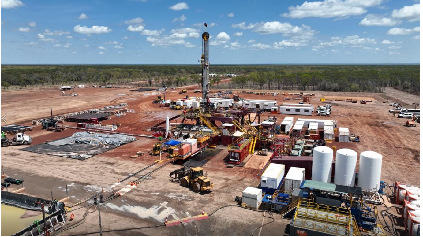
Figure 2: Drilling of Amungee 2H well on the Amungee well pad in EP 98.
