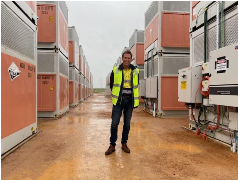
Figure 3 TMT Business Development Manager Jason Barnett at the Yadlamalka Energy Project. Source: Technology Metals Australia
