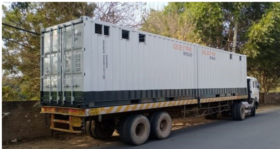
Figure 2: Delectrik VRFB ready for dispatch to USA and Australia
