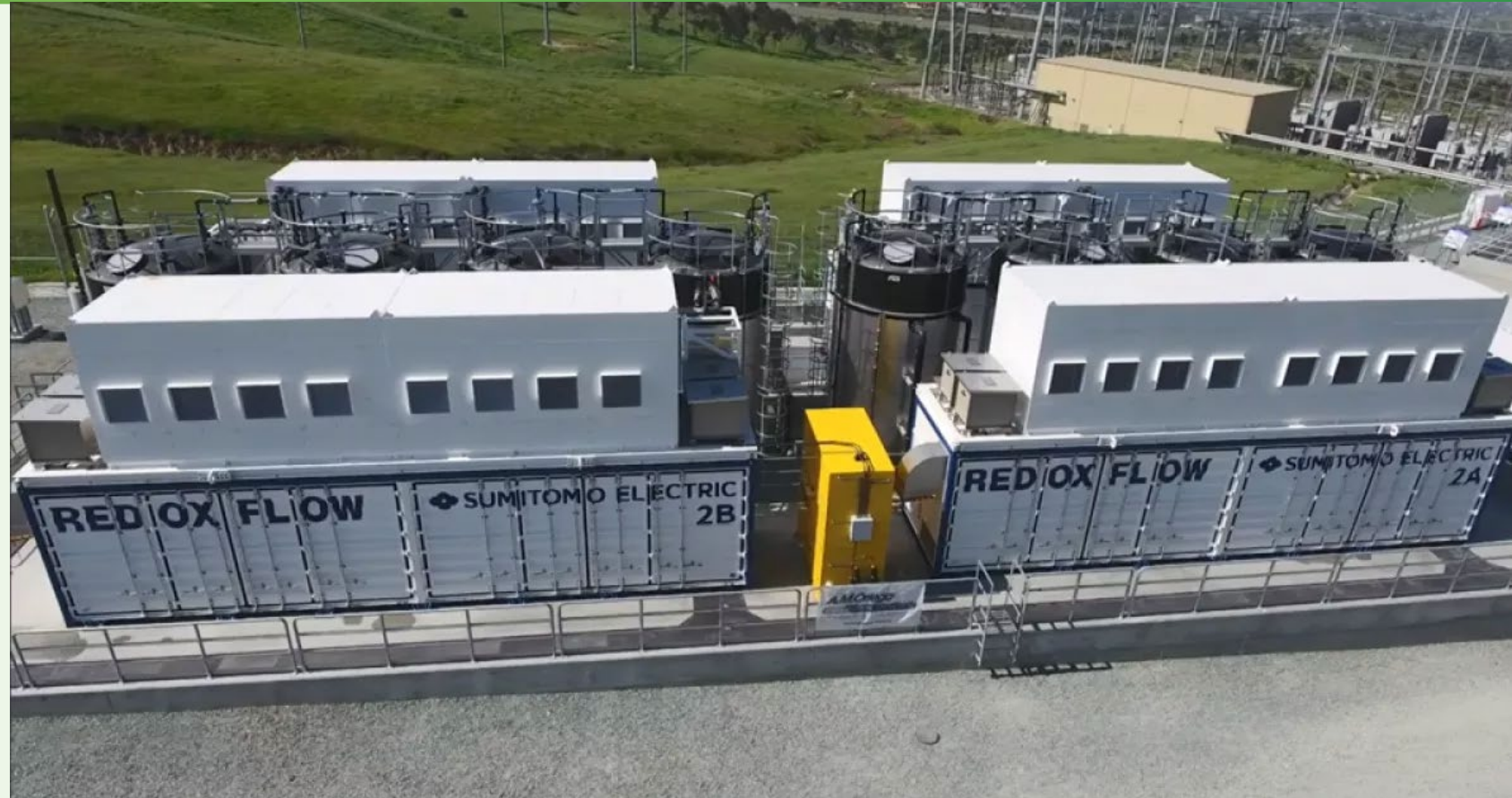
Sumitomo Electric's vanadium redox flow batteries deployed at a San Diego Gas and Electric substation in Bonita, San Diego, California. These flow batteries provide 2 megawatts and 8 megawatt-hours of energy to California's grid — enough to power about 1,000 homes for up to four hours. Source: The San Diego Union-Tribune, 28 January 2021
