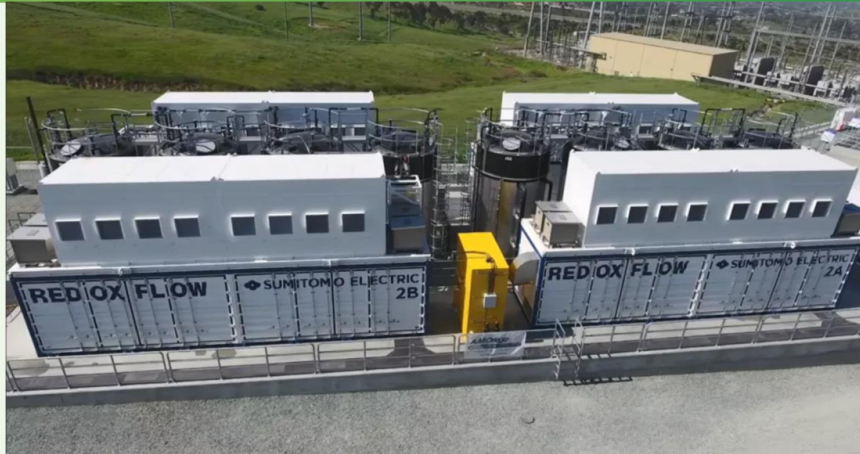
Sumitomo Electric's vanadium redox flow batteries deployed at a San Diego Gas and Electric substation in Bonita, San Diego, California. These flow batteries provide 2 megawatts and 8 megawatt-hours of energy to California's grid — enough to power about 1,000 homes for up to four hours. Source: The San Diego Union-Tribune, 28 January 2021
