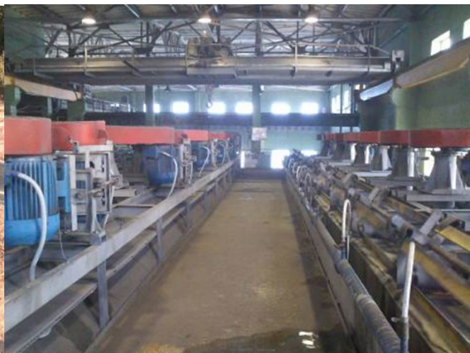
Final stage flotation cells
