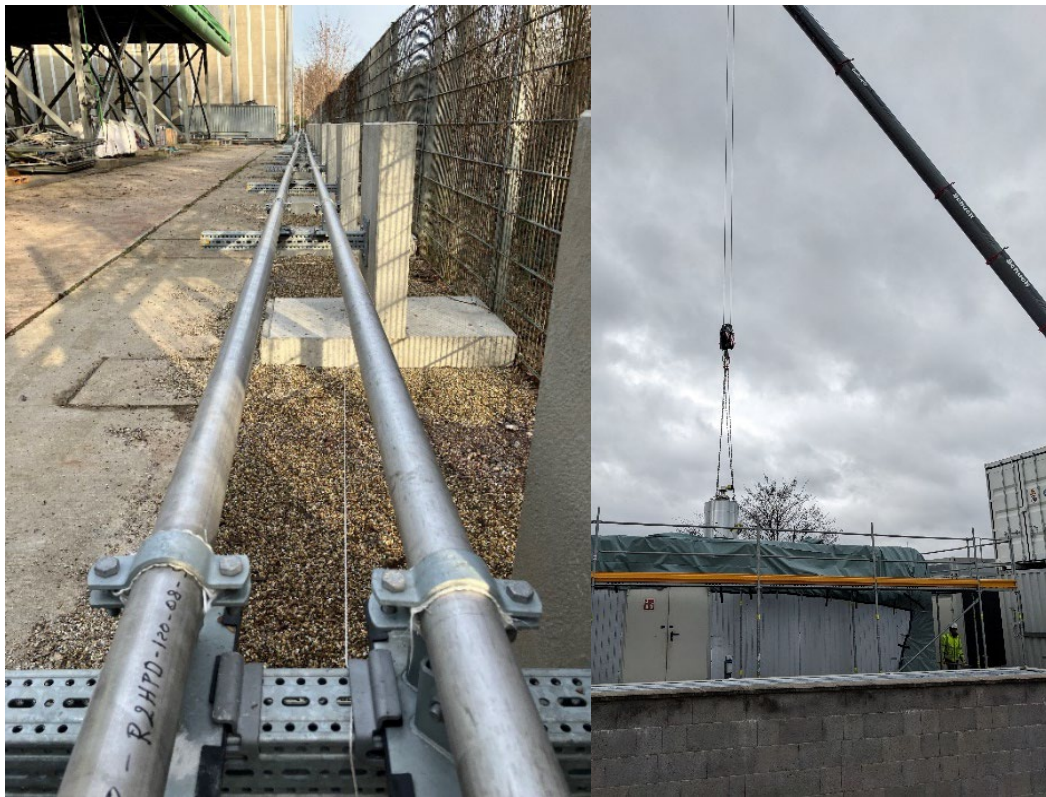
Figure 1: Brine line installation and construction progress at Vulcan's Lithium Extraction Demonstration Plant at Landau
