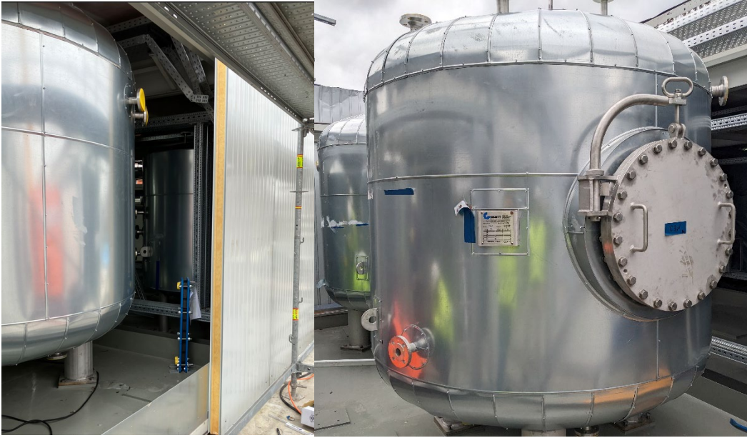
Figure 1: Brine preparation tank at Vulcan's Lithium Extraction Demonstration Plant at Landau
