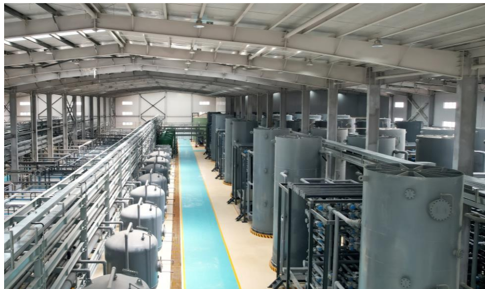
CHINA - EVEBATTERY 10,000 TPA LCE COMMERCIAL PLANT BUILT WITH SUNRESIN
