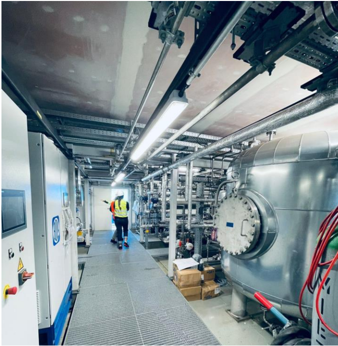
Figure 4 Water Storage tank from Water preparation system
