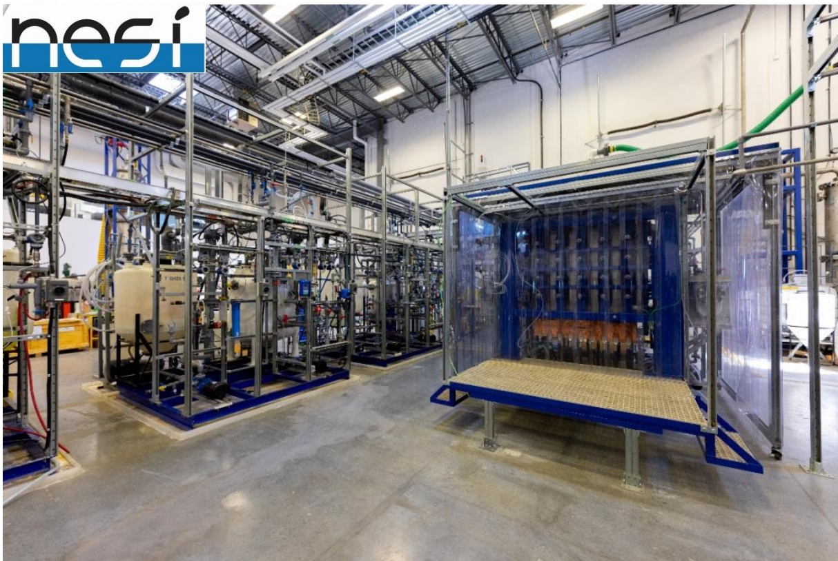
Figure 36 NORSCAND ® Cell Test setup at NESI's BC Research electrochemical demonstration plant facility in Vancouver.
