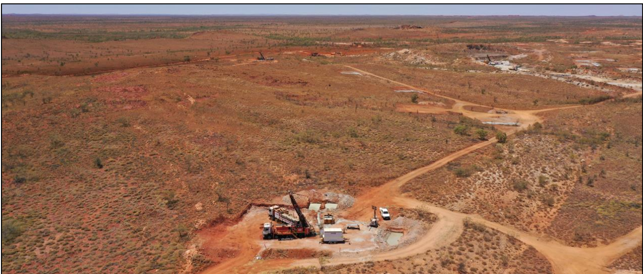
Figure 1 – Drilling at the northern end of Leia (Leia off photo to the right). View looking to the southeast.
